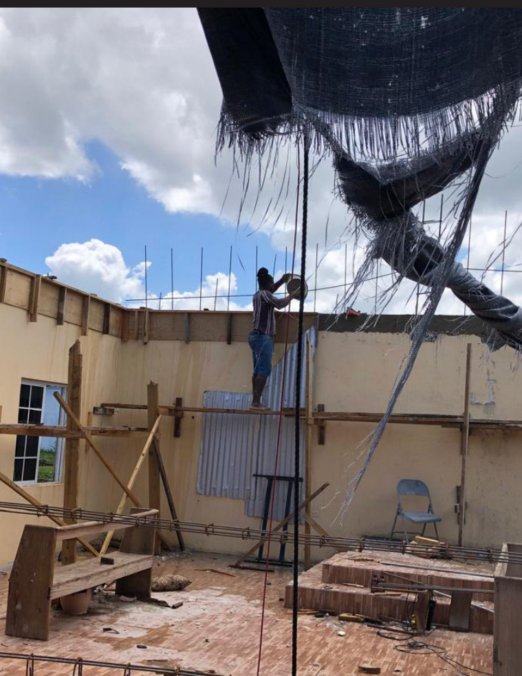
SLIPE, ST. ELIZABETH - DESTRUCTION
