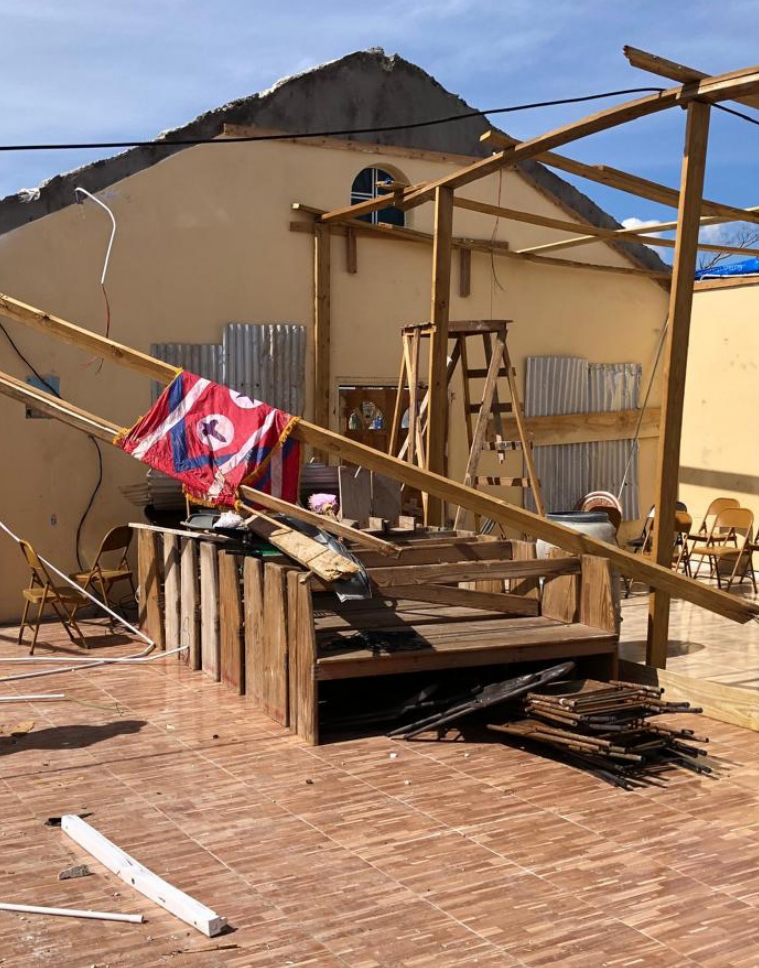
SLIPE, ST. ELIZABETH - DESTRUCTION
