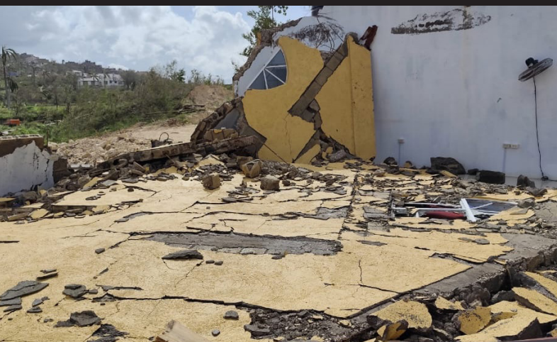
MONTEGO BAY, ST. JAMES - DESTRUCTION
